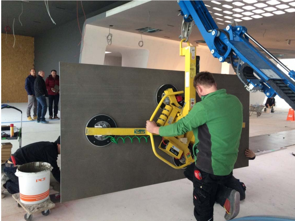
Fig. 4: To protect the health of his team and to ensure high-quality tile laying, master tiler Hansjürgen Kulmer used a tile laying crane.
